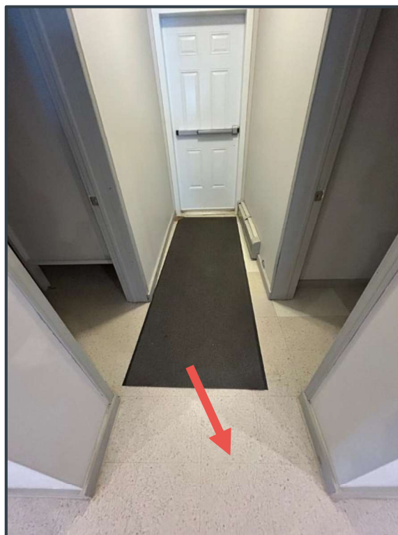
Photograph 8: Asbestos-containing 12" x 12" (30cm x 30cm) beige with black specs vinyl floor tiles in the Municipal Complex Hallway (Englobe Sample ID: 09A-C)
