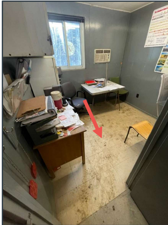
Photograph 2: Asbestos-containing 12" x 12" (30cm x 30cm) beige with red streaks vinyl floor tiles in the Public Works Garage Office (Englobe Sample ID: 02A-C)
